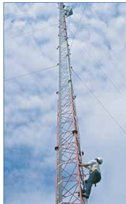
LAD-SAF® Kit installed on a tower
